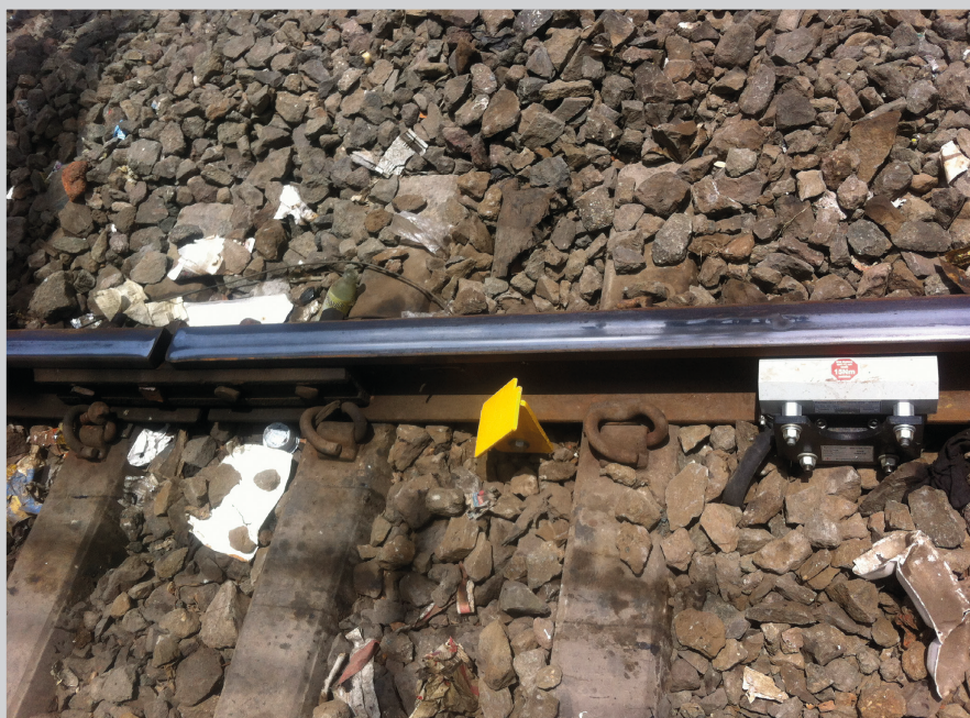
Figure 2: Conditions rendered more difficult by inadequate track maintenance.
