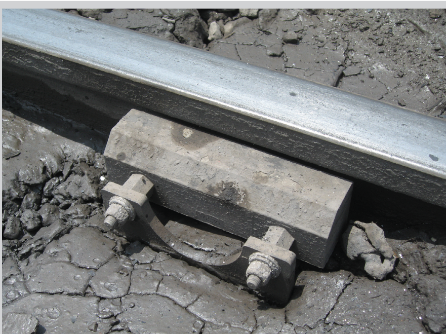
Figure 5: Floods leave long-term damage.
